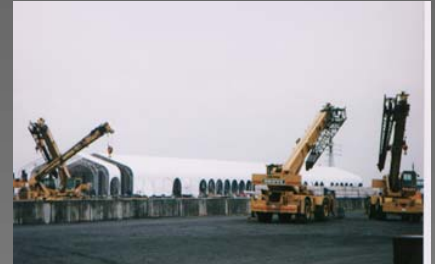
CAMSS60EX being used as a temporary building during steel plant construction on Lake Michigan.
